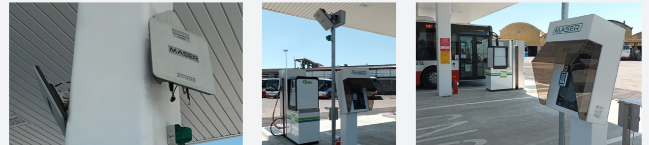
Illustrations: The RFID readers have been mounted facing downwards directly above the gas pump and thus enable accurate and automatic vehicle identification. This has led to significant acceleration of the refueling process and has provided data on refueling frequency and energy costs for controlling purposes.
