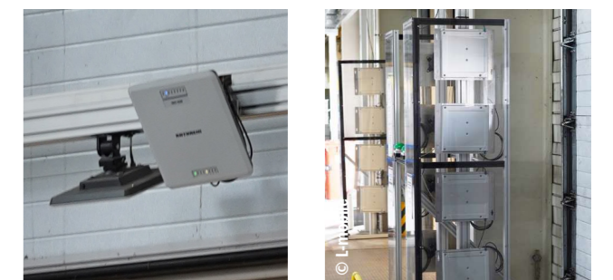
Figure: the KATHREIN RRU 4500 readers were installed directly above the loading gate, and the SSMH antennas to the side of the gates to capture the tagged parcels.
